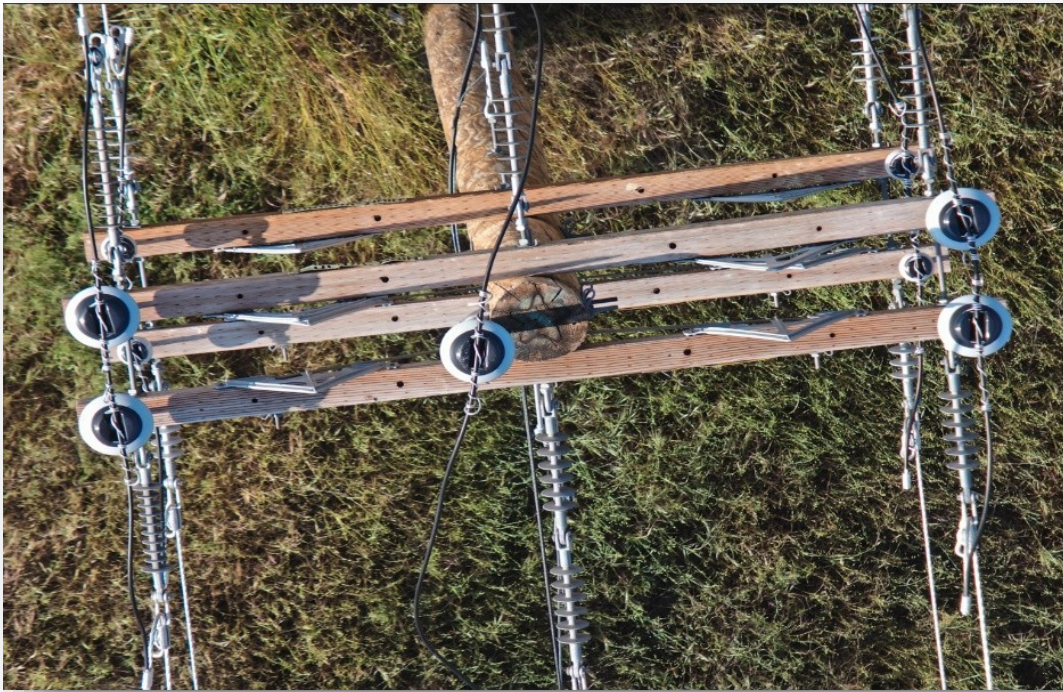
Figure 14 – Drone Photo of a Distribution Pole
