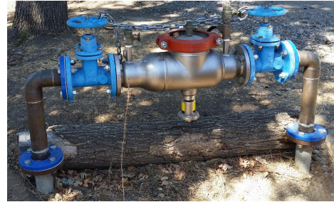
Example of a Backflow Prevention Assembly
