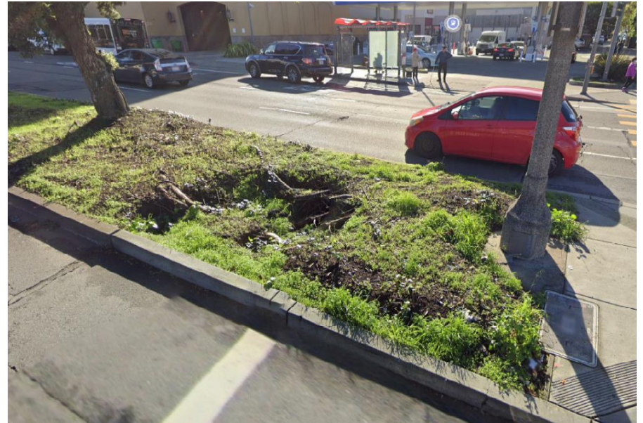
Sinkhole at Geary Blvd and Arguello Blvd in October 2023
