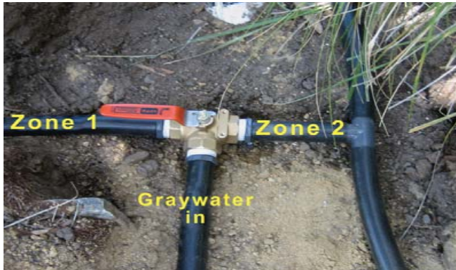
This 3-way valve creates two zones in the landscape. Water can be redirected from one zone to another zone by turning the handle. Photo: Laura Allen.
