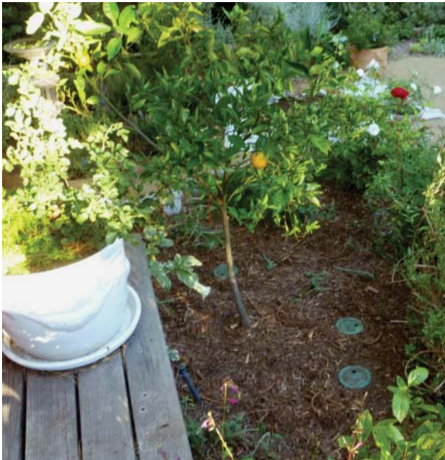
This graywater system is used to irrigate plants with similar water needs. The fruit trees and larger perennials are irrigated from the laundry machine in one “hydrozone.” Photo: Leigh Jerrard.
