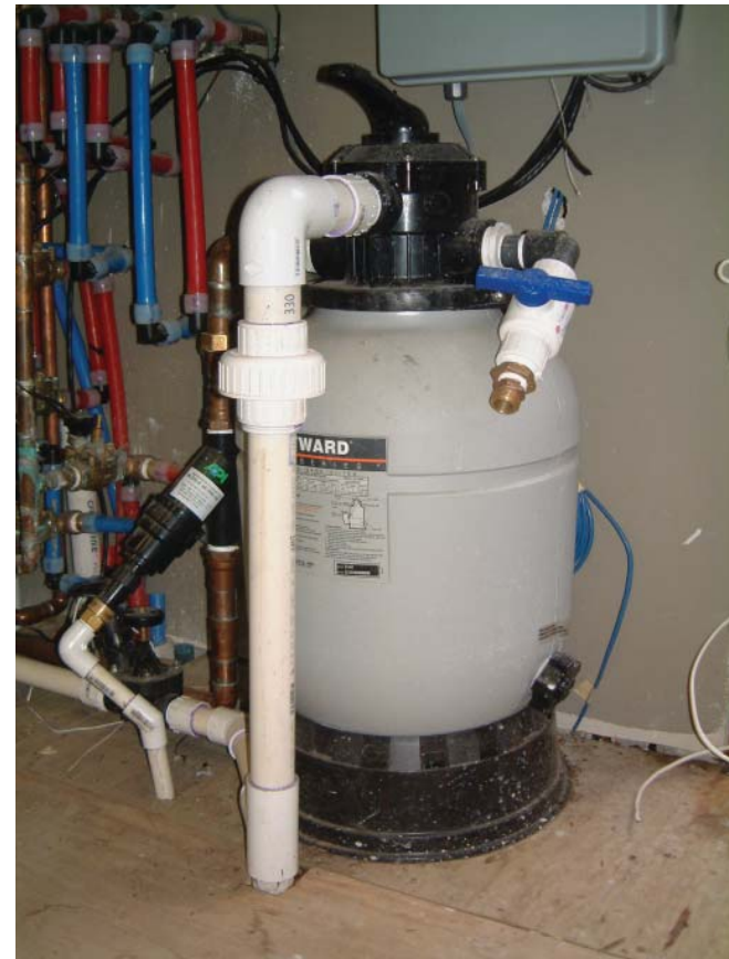
Graywater filter at the Sunset San Francisco Idea House. Photo: WaterSprout.
