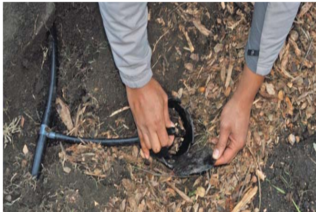
Adjusting flow by rotating the tees. Ball valves can be added to the ends of small tubes, if necessary. Photo: David Glover.
