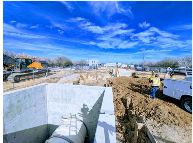
San Joaquin Pipeline Valve and Safe Entry Newly Backfilled Removable Spool Piece Vault at Pelican Valve House, Prior to Lids being Installed
