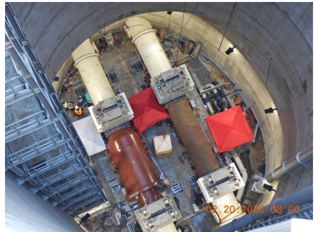
Mountain Tunnel Improvements Project: Priest Flow Control Facility Shaft with two 72-inch diameter pipes, four Knife Gate Valves, one Sleeve Valve and One Spool Piece
