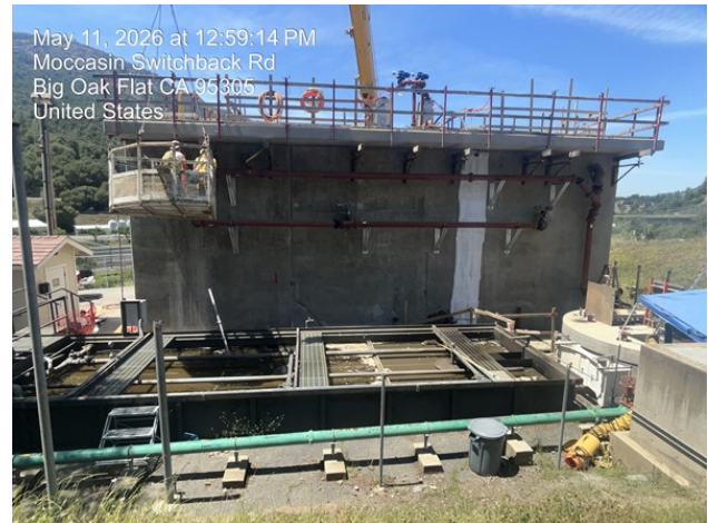
Moccasin Wastewater Treatment Plant Sequential Batch Reactor Structure
