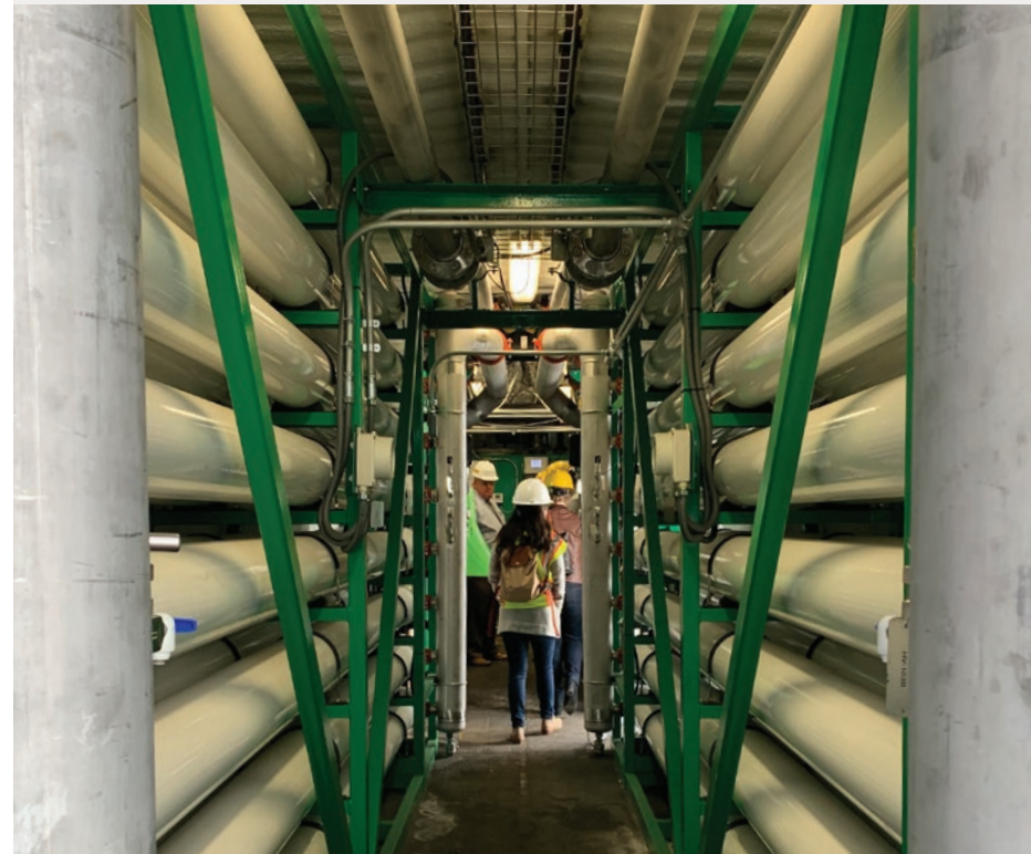
Energy Center San Francisco's closed circuit reverse osmosis system (image courtesy of SFPUC)
