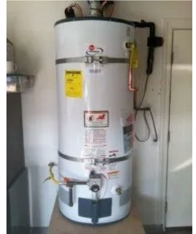
Existing Equipment Photo
