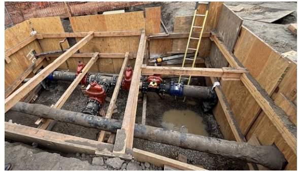
New Town of Sunol Pipeline Interconnection
