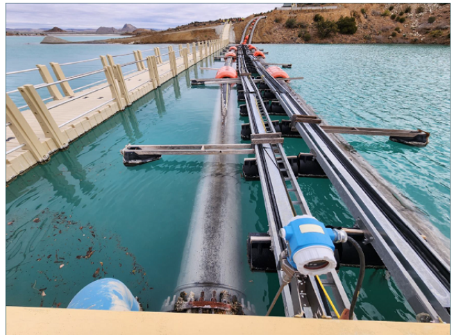
Barge Pump Example at Mining Facility
