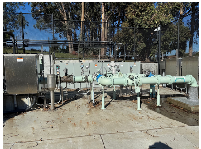
Pump Running During 5-Day Testing at Colma Blvd Well Station
