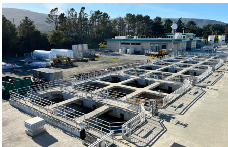
HTWTP filter beds
