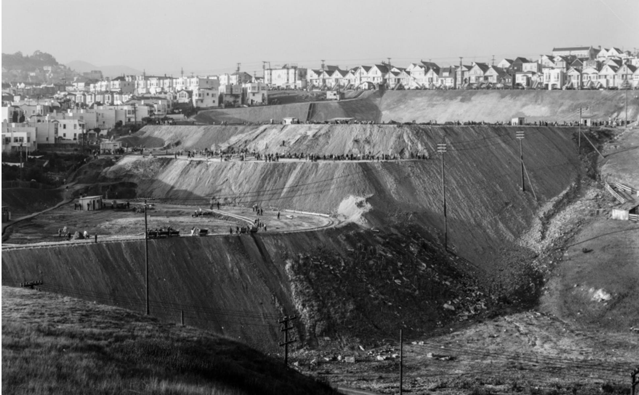
Construction activity on St Mary's Park (above), view toward Alemany Blvd from St Mary's Park (reverse) source: OpenSFHistory / wnp14.2793 (above), wnp36.03380 (reverse)
